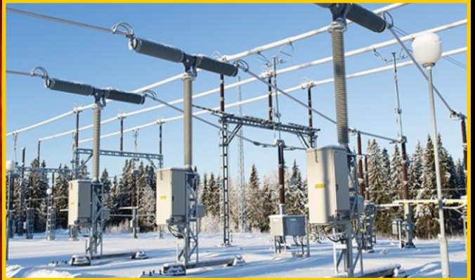
Substation Structures Power
